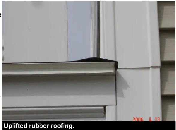
Uplifted rubber roofing.
