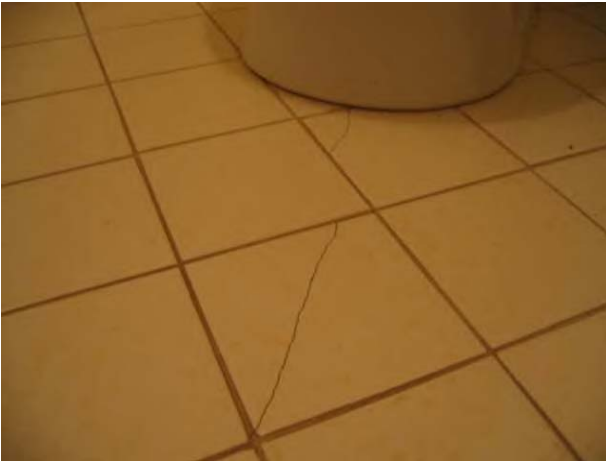
Cracked floor tiles
