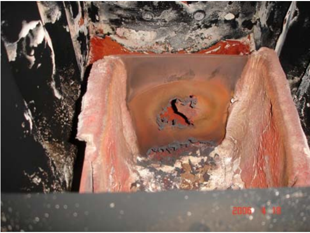
UNSAFE. Hole burned through fire chamber
