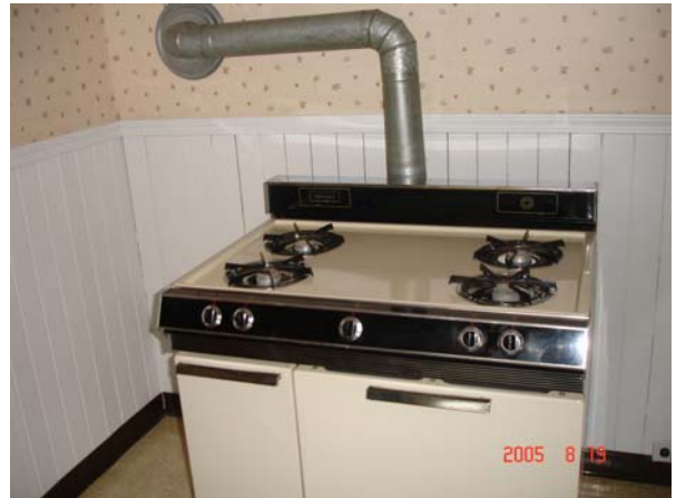
Improper pitch @ flue pipe
