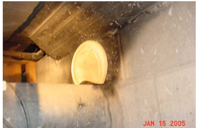
UNSAFE old flue opening
