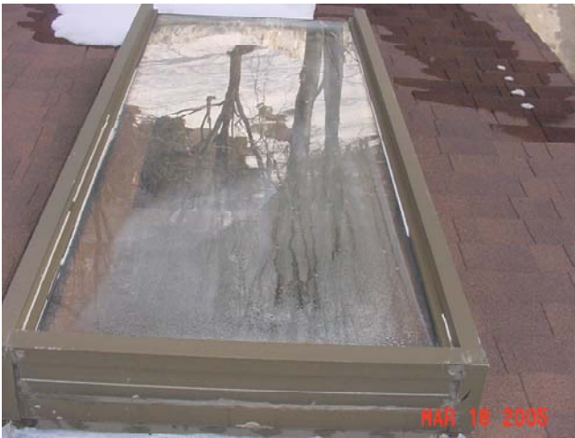
Faulty glass skylight glass
