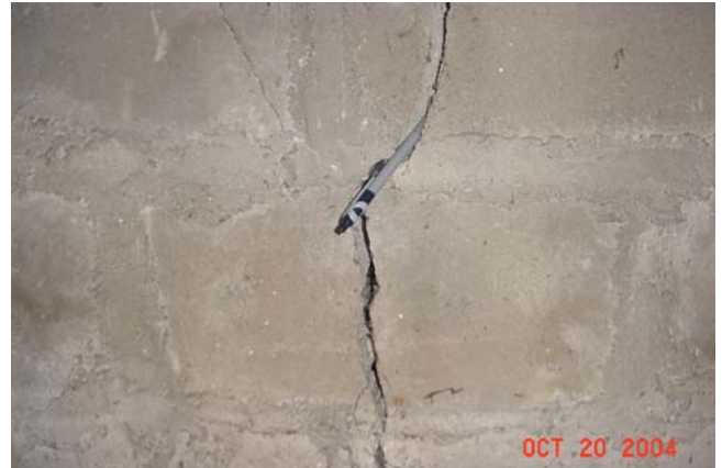
Crack in foundation
