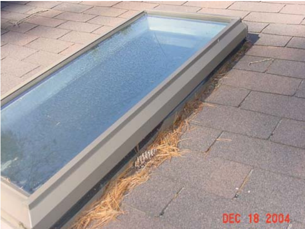
Foggy glass @ skylight
