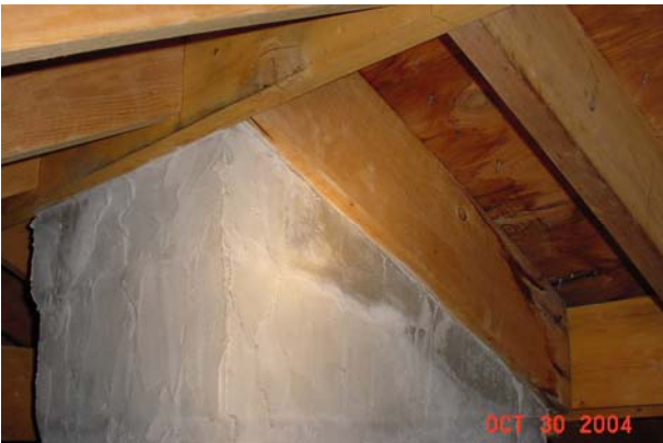
UNSAFE, wood against chimney
