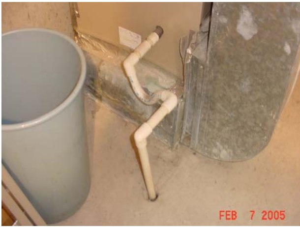
Condensate drain under floor
