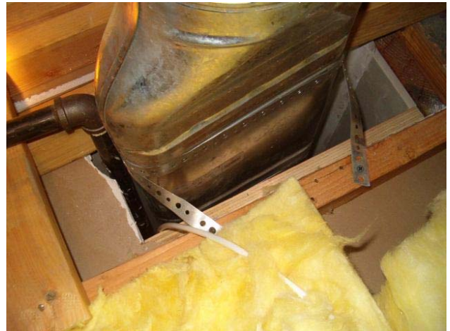
UNSAFE, missing firestopping
