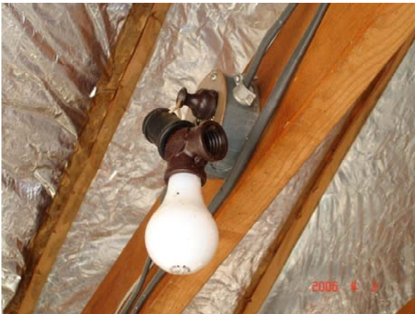
Unsafe light fixture
