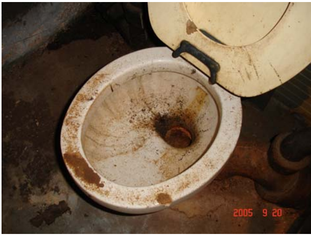
Abandoned toilet – dry trap
