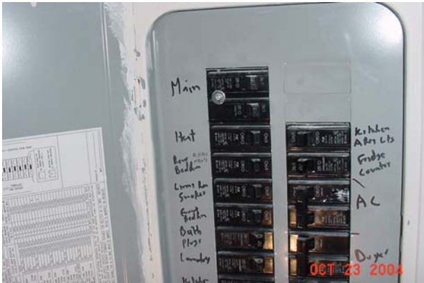
Missing link @ main breaker
