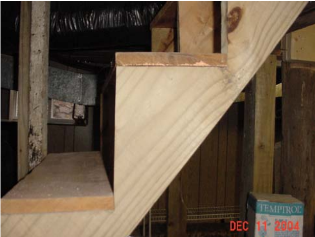
UNSAFE stair construction
