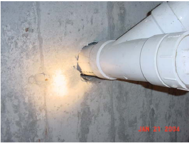
Pipe penetration hole not sealed
