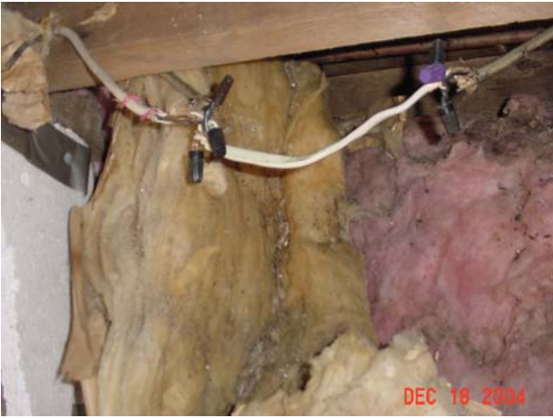
Open electrical splice
