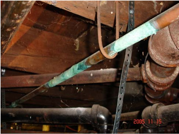
Corroded water pipe
