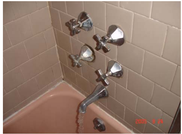
Obsolete valve assembly
