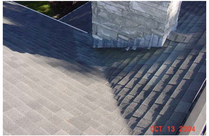
Drainage choke point, blocked valley
