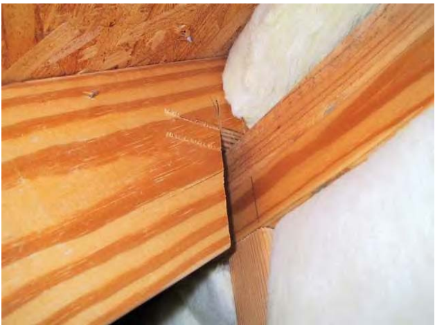
Over-notched roof rafter
