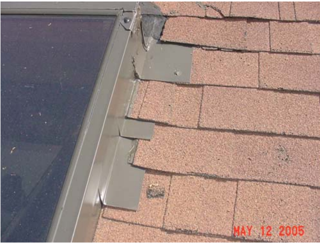
Faulty skylight flashing
