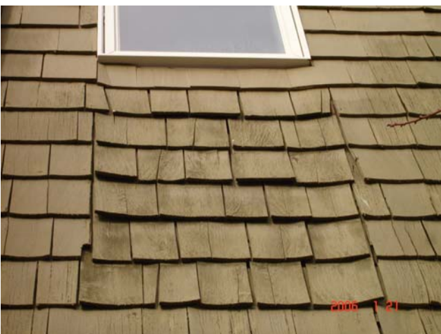
Amateur siding alterations
