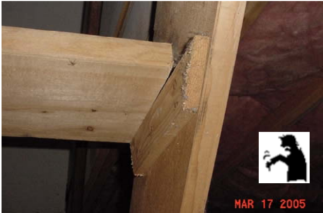
BASEMENT STAIRS. ONLY TWO STRINGERS & NO LEGS
