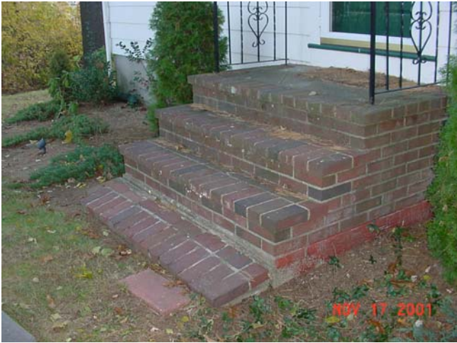
Broken / settled tread, Unsafe steps
