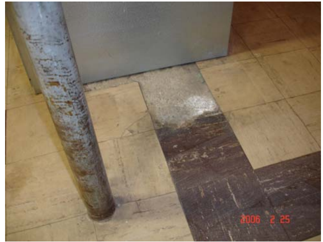
9 x 9 tiles may contain asbestos
