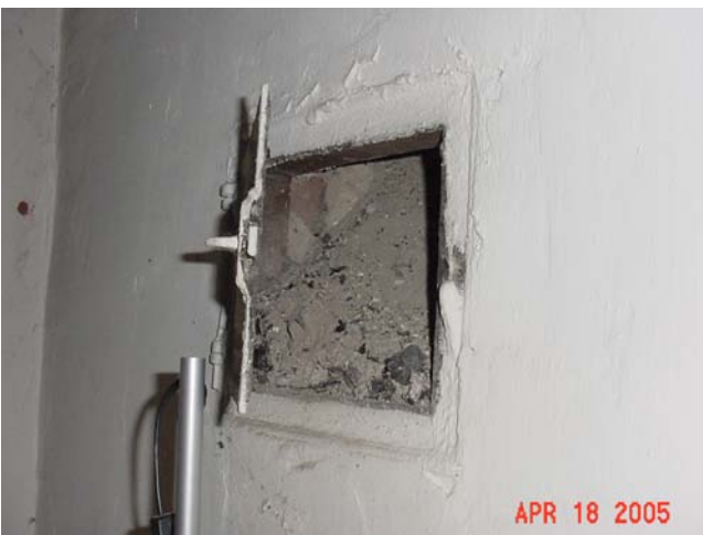
Chimney flue full of ashes
