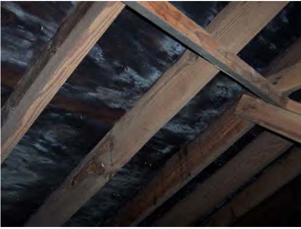
Suspected black mold in the attic
