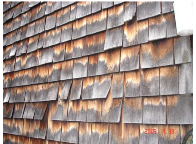
New siding needed
