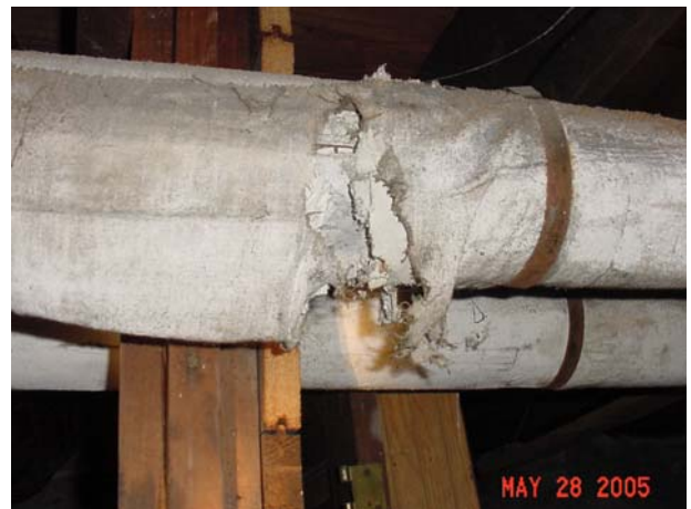
UNSAFE – friable asbestos
