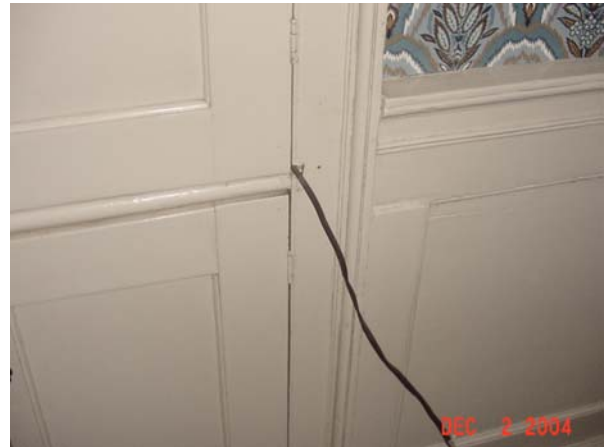
FIRE hazard. Extension cord through door
