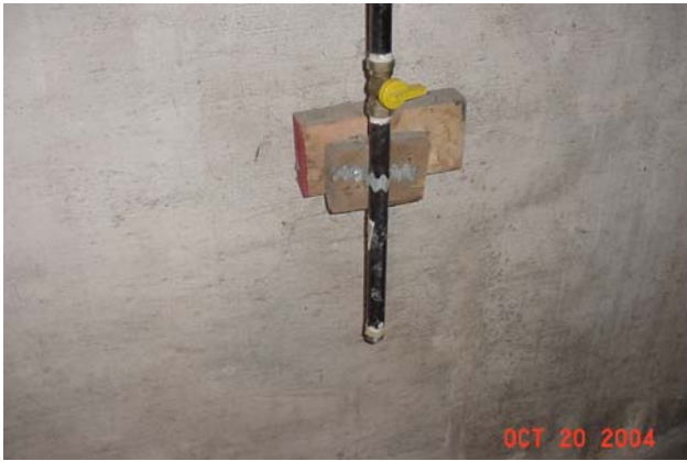
Missing cap on gas line
