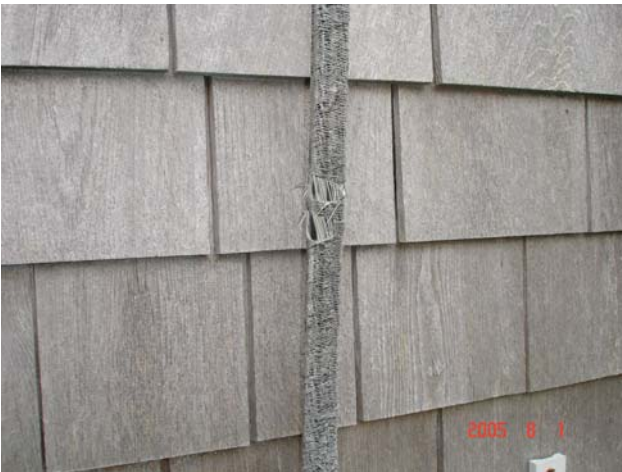
Frayed service cable
