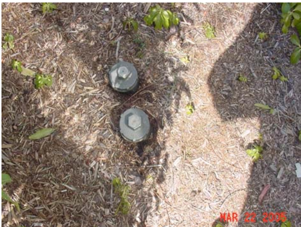
Underground oil tank found
