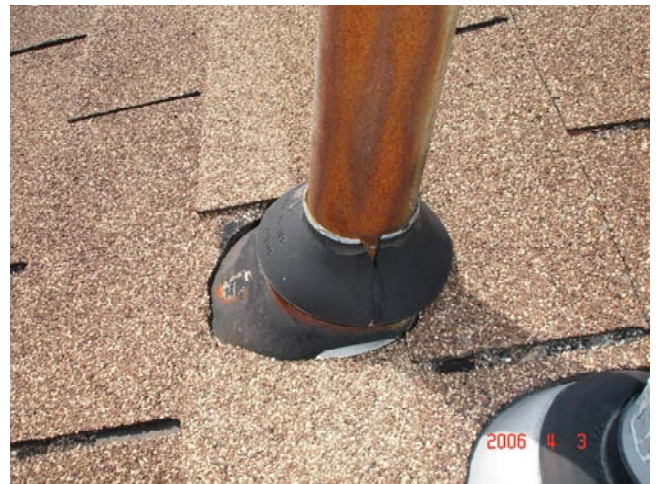
Defective rubber gasket
