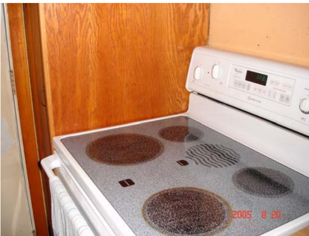
No clearance to combustibles
