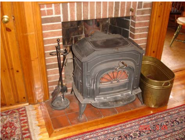
UNSAFE fire clearances
