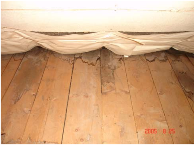
Water stains on eaves floor
