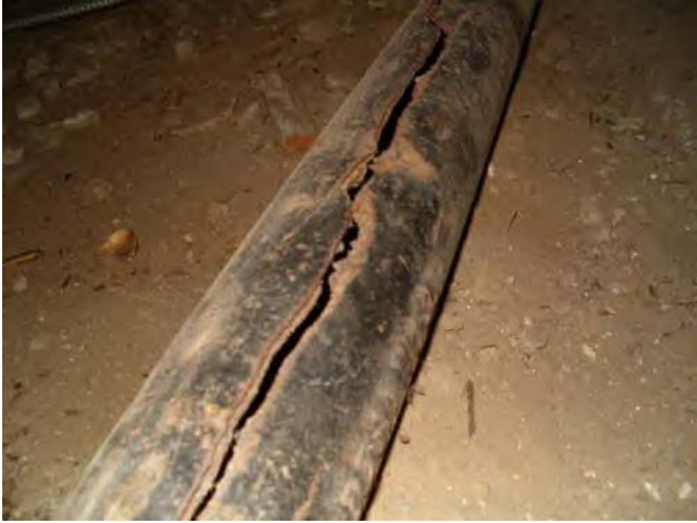
Cracked waste pipe
