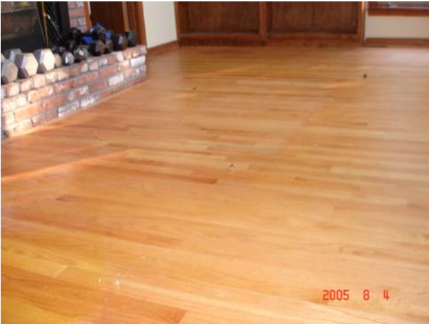
Floor not level
