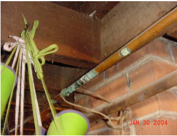
Corroded water pipe
