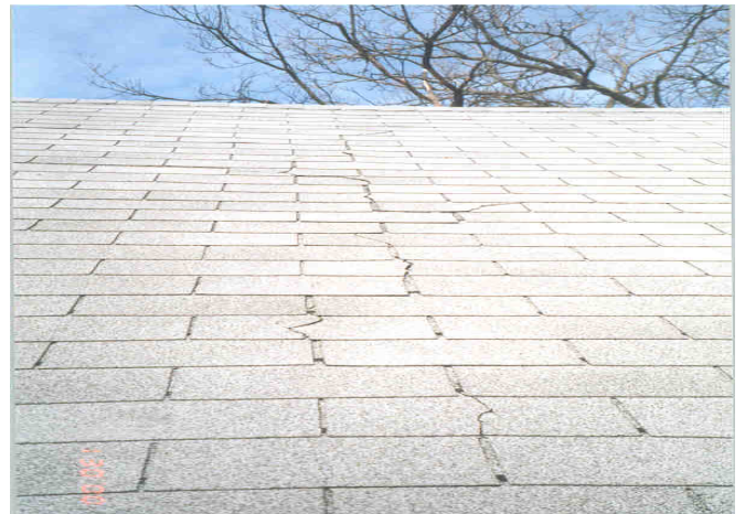
Defective, cracked shingles
