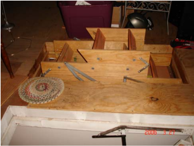
No firewall between condo attics
