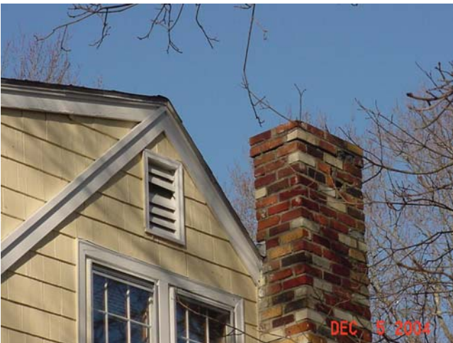
Chimney not high enough
