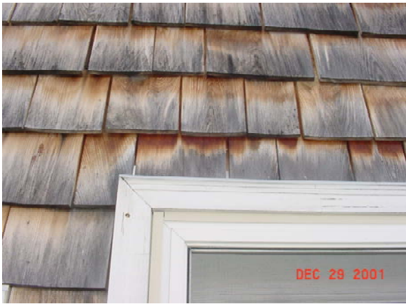
Flashing leaks above window
