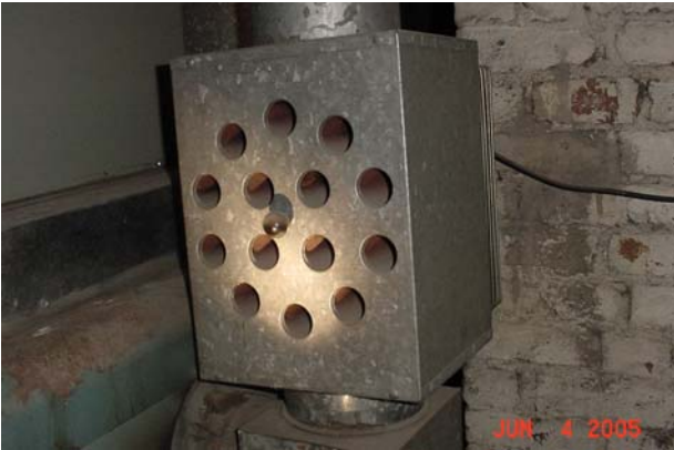
Beware of 2 nd heat exchanger
