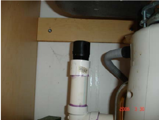
Amateur vent under sink
