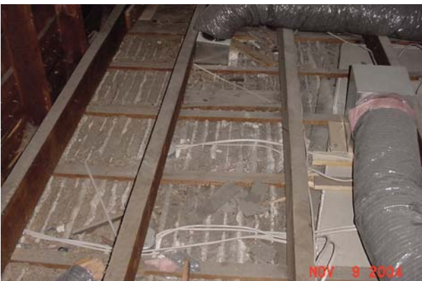
No attic insulation
