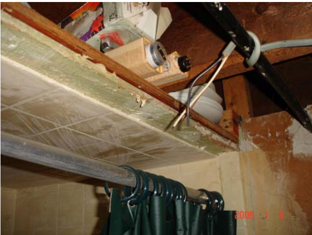
UNSAFE, live wire above shower stall
