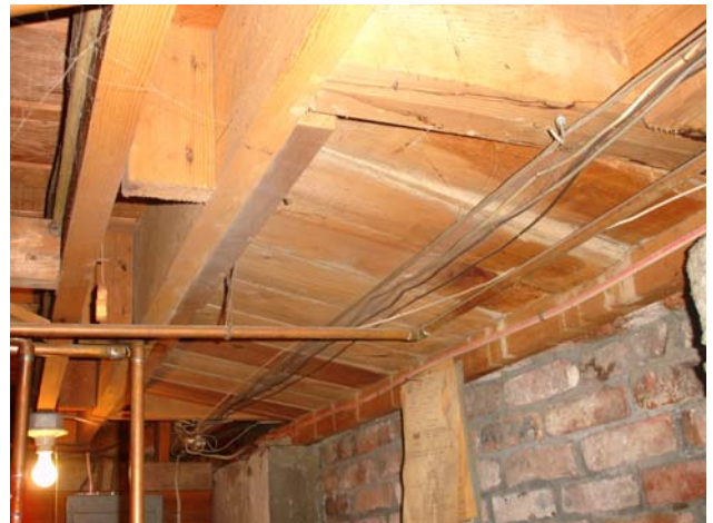
Combustible forms left under hearth extension
