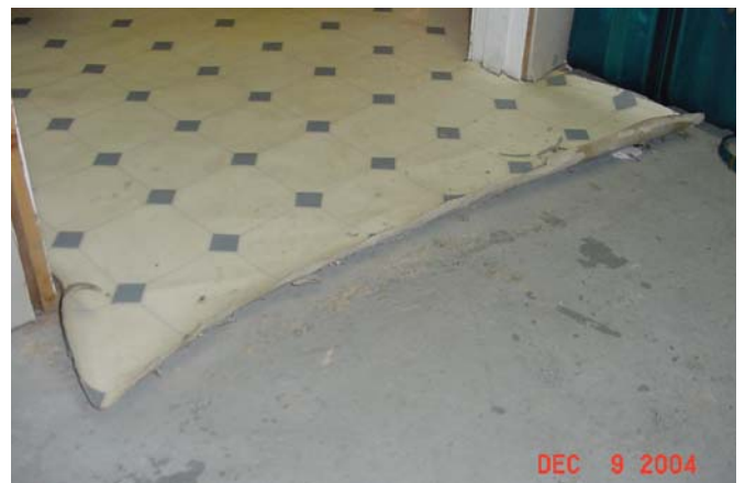
Unsafe floor covering
