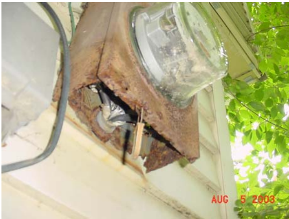
Rusted out meter box
