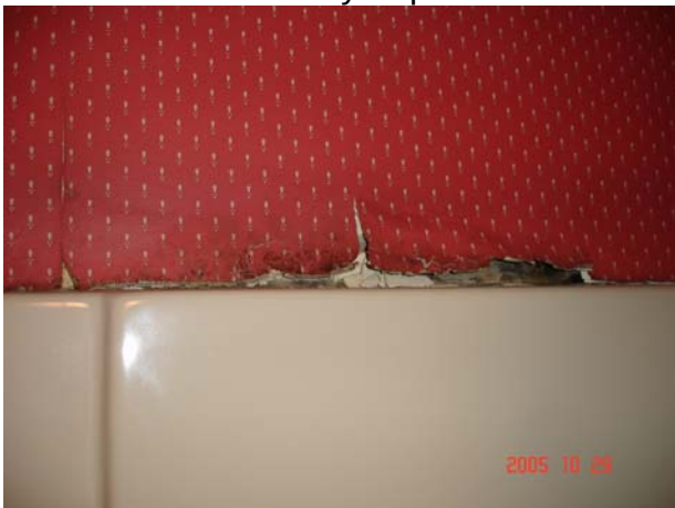
Suspected mold in bathroom
