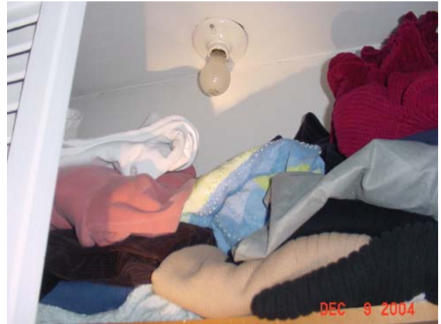
Bulb in closet = fire hazard
