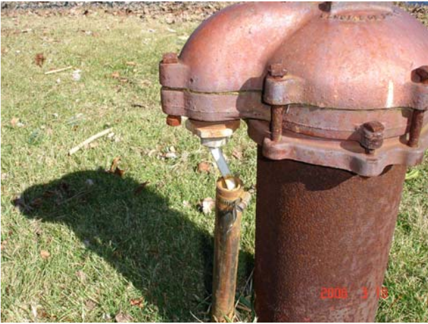
Broken wiring to well
