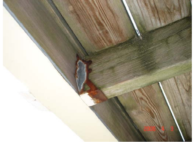
Rusted deck joist hangers
