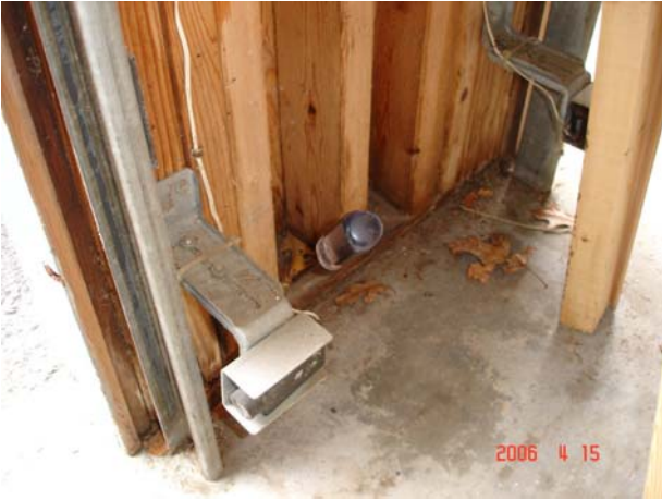
Termite decayed sill
