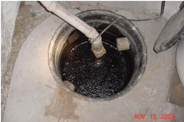
Oil in sump
