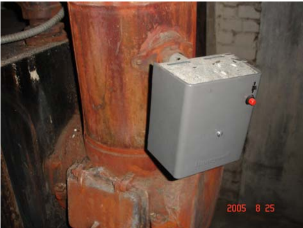
Obsolete primary control
