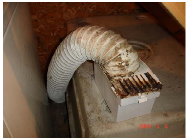
Dryer vent is a fire hazard
