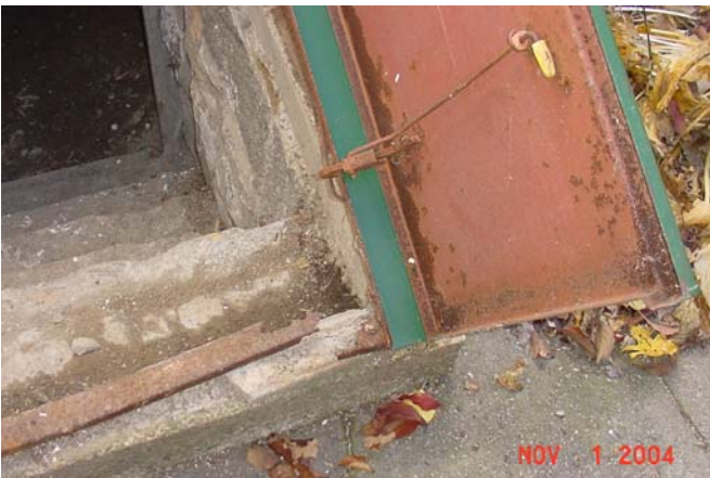
Rusted out bulkhead
