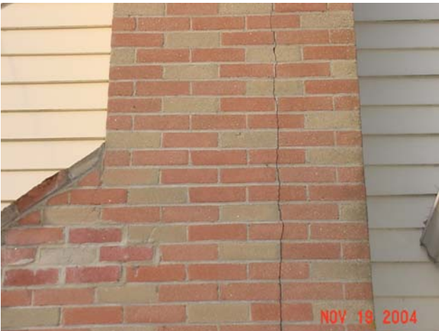
Cracked fireplace chimney
