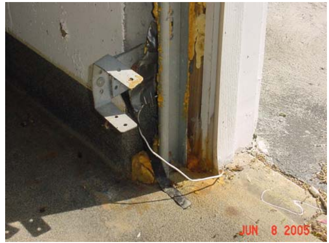
Photo sensor broken off
