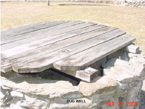
UNSAFE cover on dug well
