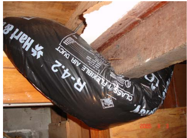
Poorly run flexible duct
