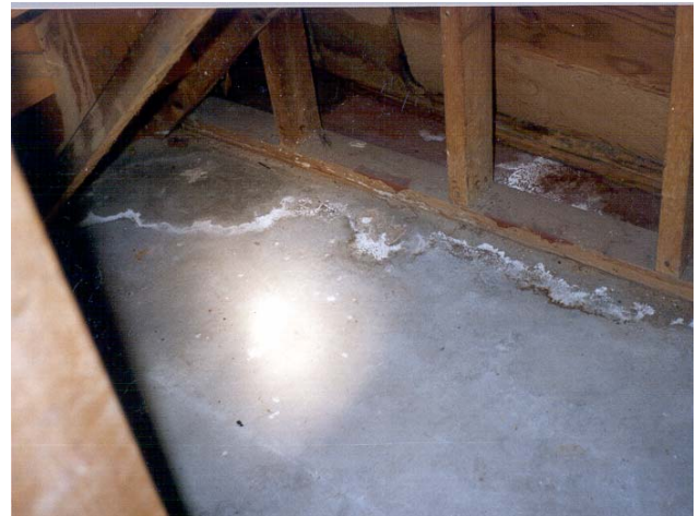
Water stains in basement
