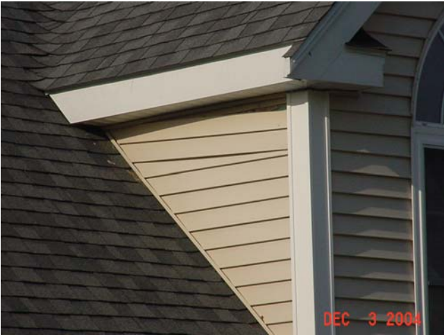
Loose vinyl siding
