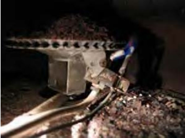
Water heater burner
