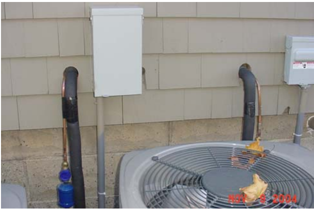
Disconnect behind AC
