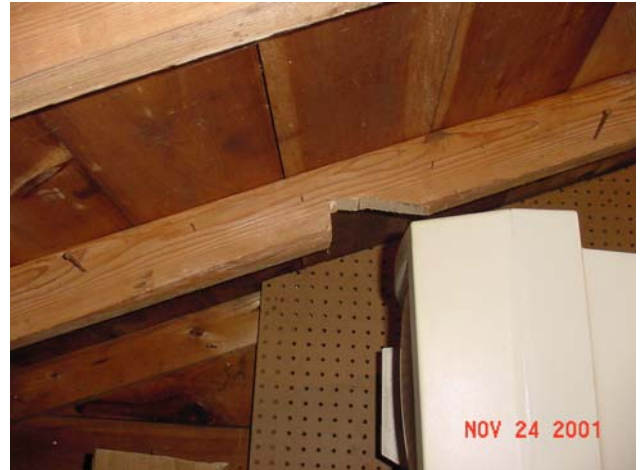
Notched roof rafter
