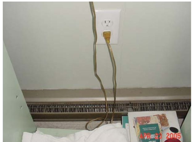
UNSAFE, outlet above electric heater
