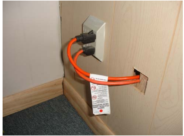
Extension cords through wall
