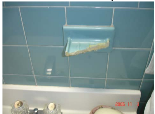
UNSAFE – broken soap tray
