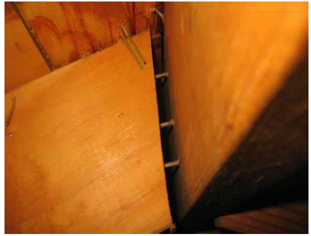
Rafter pulling away from ridge
