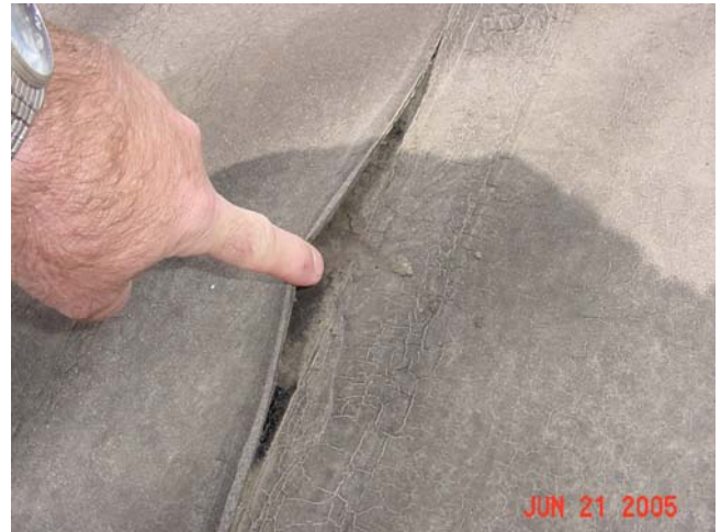
Rubber roof covering leaks
