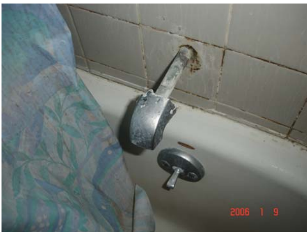
Rusted out tub spout
