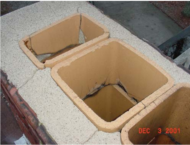
Defective flue liners
