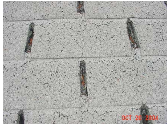
Perforated slots – replace the roof
