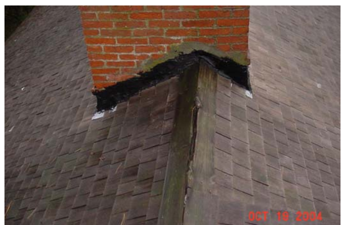
Defective ridge board
