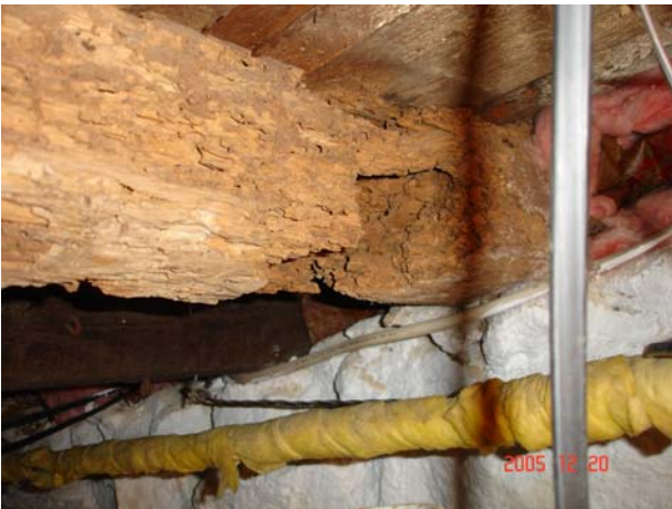
Extensive pest damage
