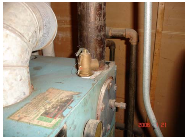
UNSAFE, missing drain pipe
