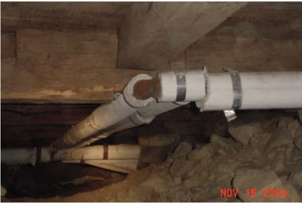
Asbestos on steam pipes
