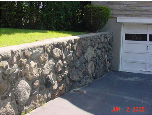
UNSAFE – missing guard railing
