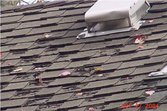
New roof needed
