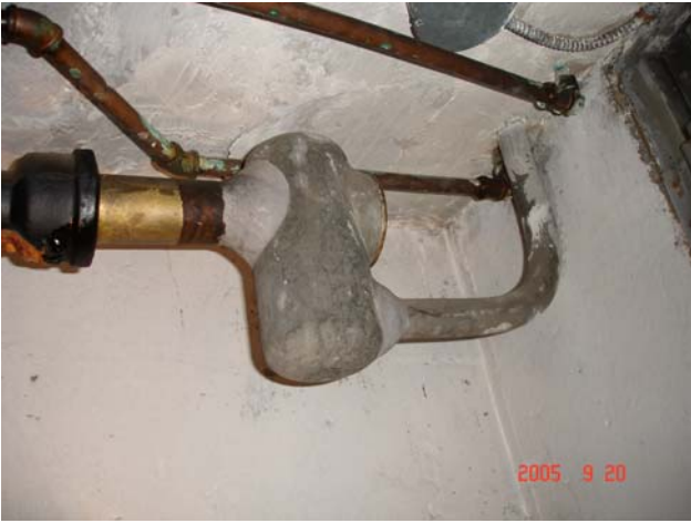
Obsolete lead drum trap
