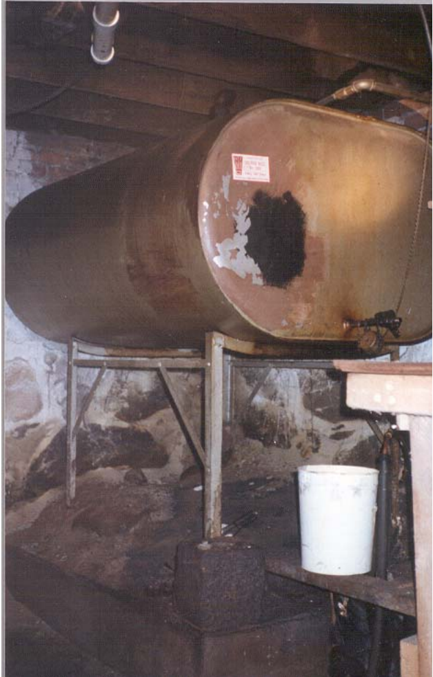
Leaky oil tank
