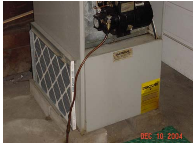
Furnace lacks return duct
