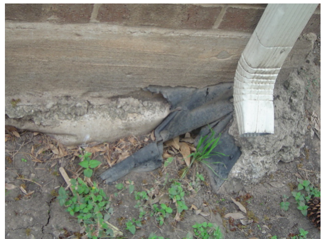
Faulty downspout causing soil erosion
