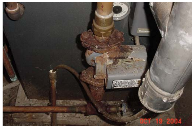
Corrosion at circulator pump
