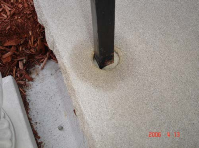
Post holes not crowned
