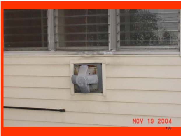
UNSAFE space heater vent
