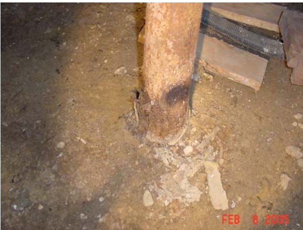
Rusted out steel column
