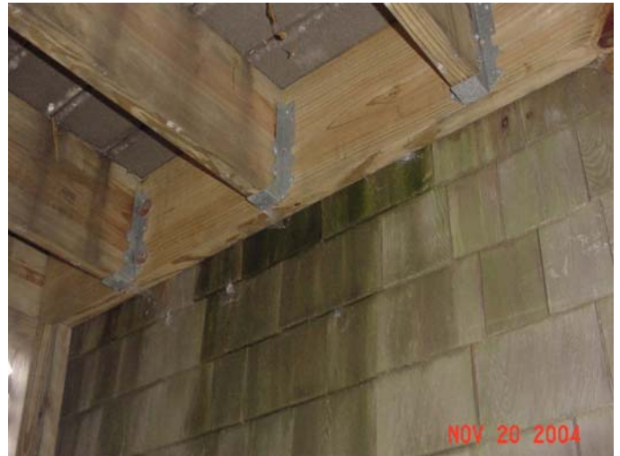
Missing flashing & lag bolts @ deck ledger
