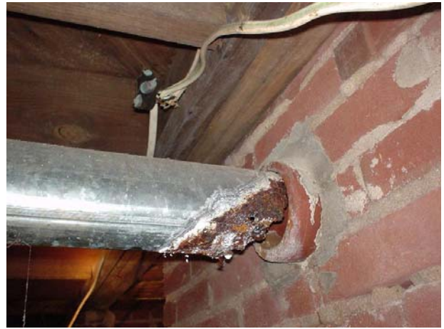
UNSAFE, rusted out flue pipe
