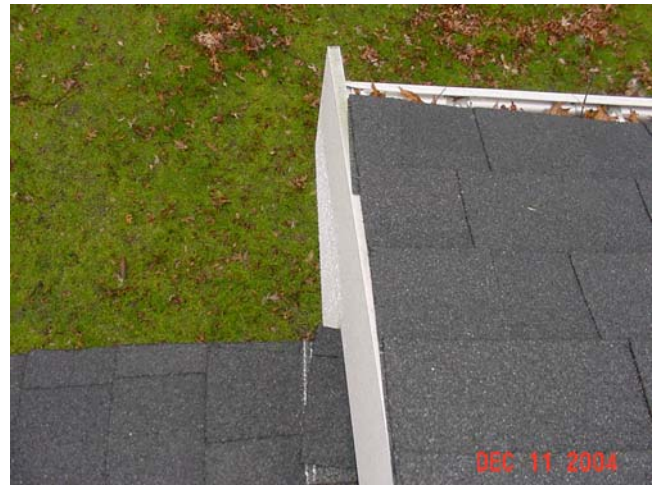
Poor workmanship at edge of roof
