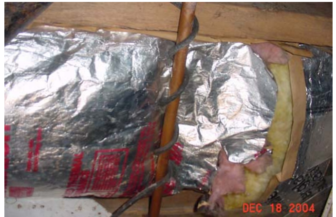
Live wire wrapped around pipe
