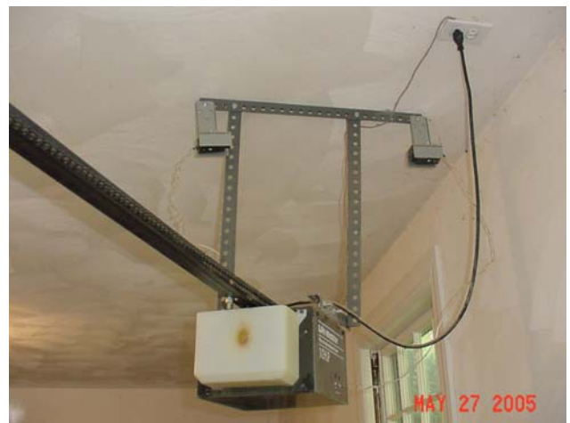
Faulty photo sensors
