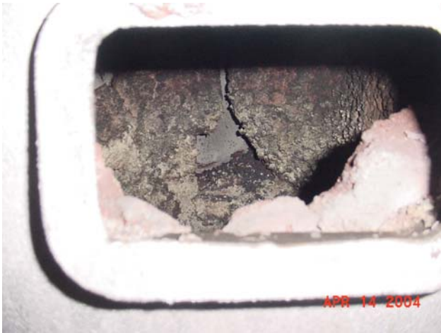
Defective fire chamber liner
