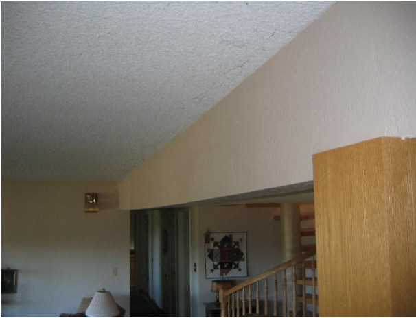
Sagging where bearing wall removed
