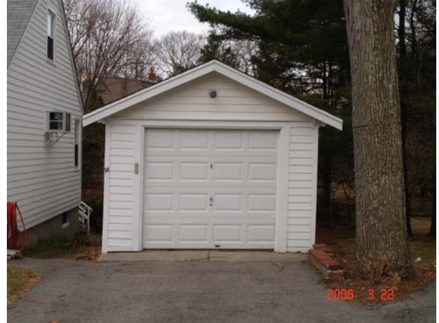
Racked or tilted garage
