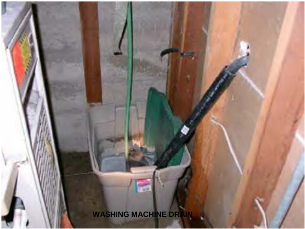
Washing machine drain
