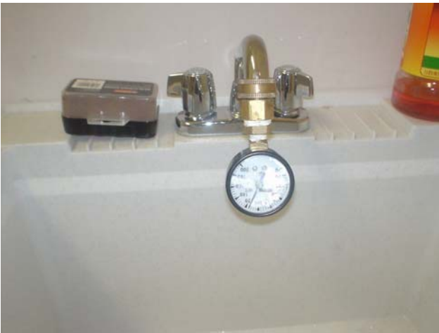
Danger, 115 psi water pressure
