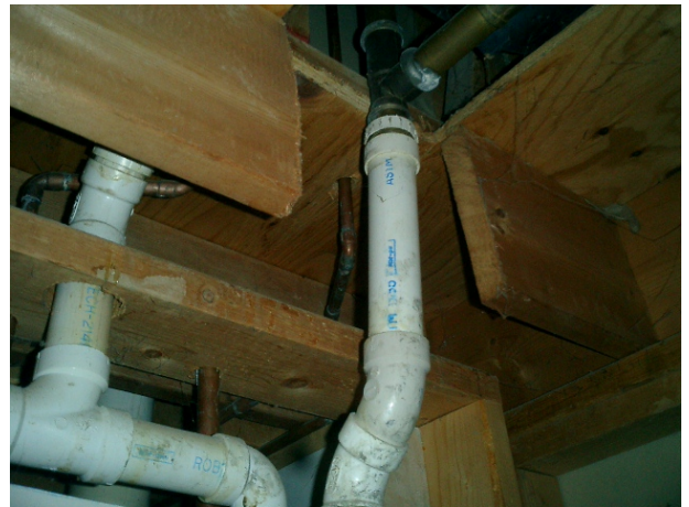
Joist cut off under tub
