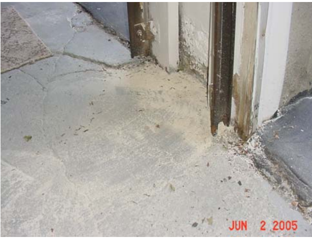
Cracked and settled concrete floor
