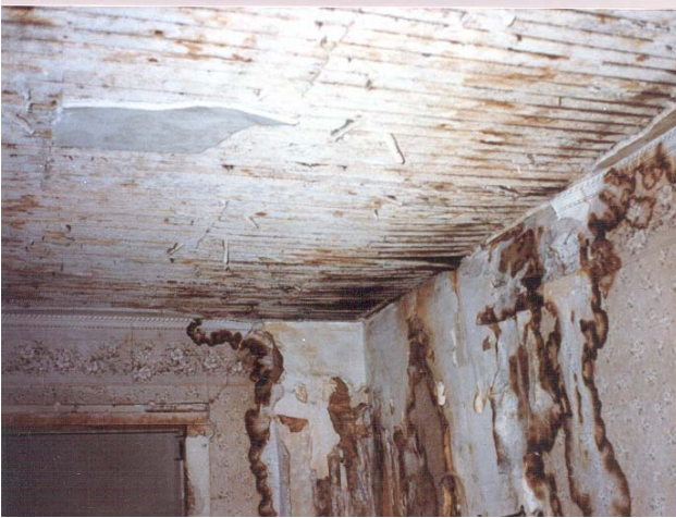
Water damaged ceiling & wall
