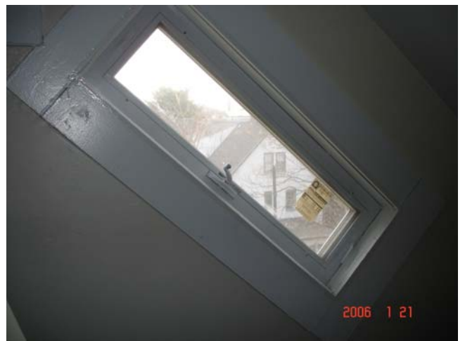
UNSAFE bedroom egress window
