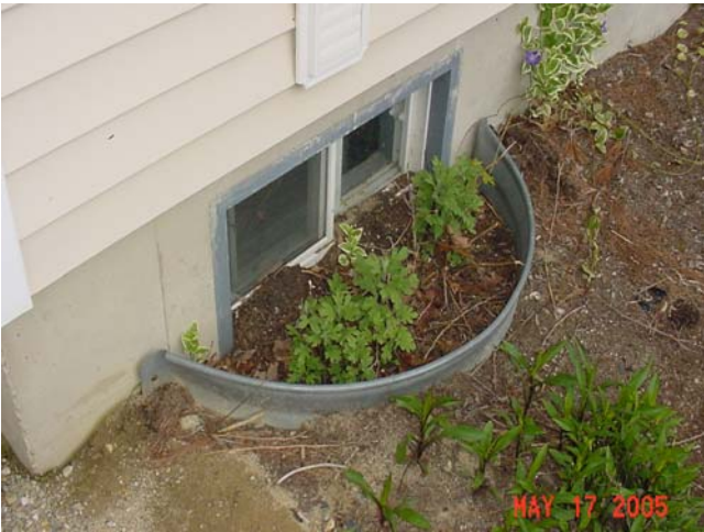
Faulty window well grading
