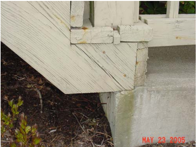
Tread lightly on UNSAFE stairs
