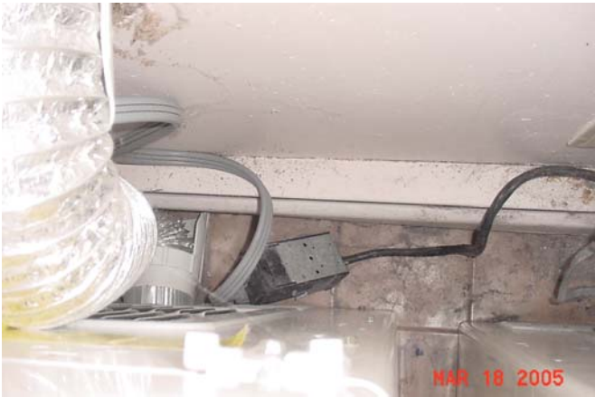
Faulty dryer duct & outlet
