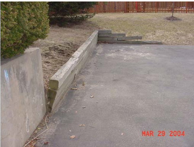
Failed retaining wall
