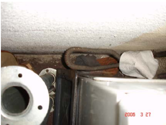
UNSAFE flexible gas line
