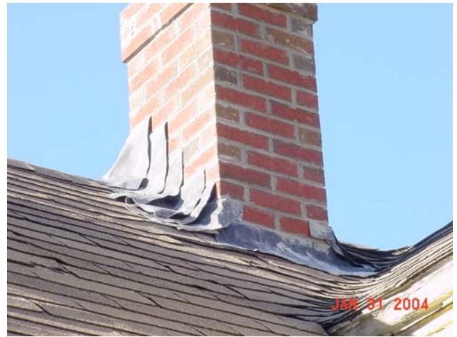
Faulty chimney flashing
