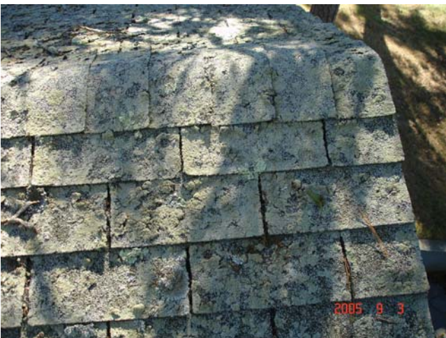
Algae covered roof
