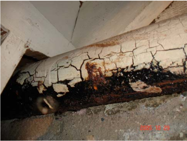
Leaking cast iron waste pipe
