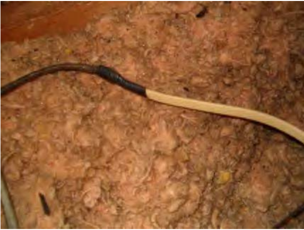
Spliced wires / no junction box
