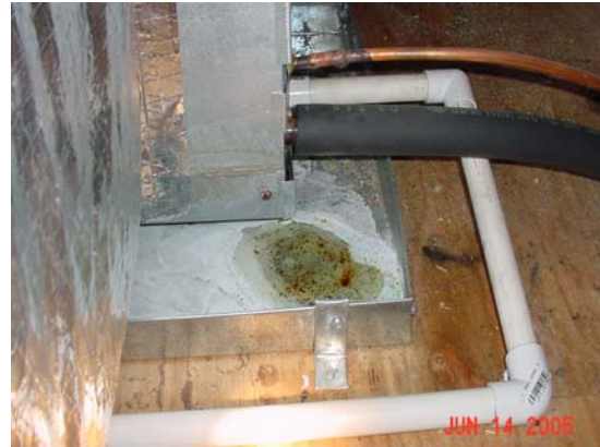
AC condensate leak in attic
