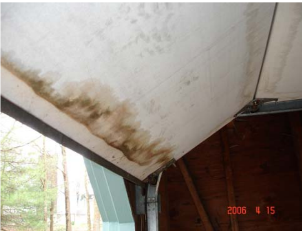
Water damaged overhead door
