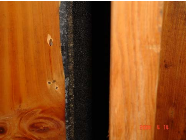
Improper ridge vent slot @ ridge board
