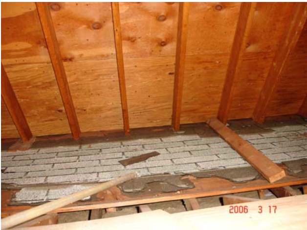
Fire hazard, old shingles not removed when an addition was built.
