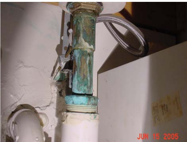
Leaks under the sink
