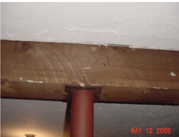
Missing fireshield on wood girder
