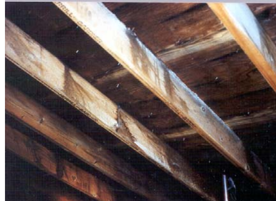
Active roof leaks
