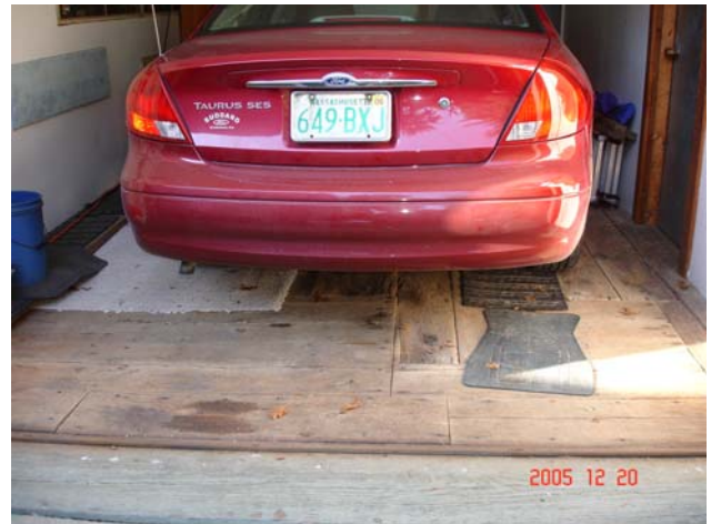
UNSAFE, combustible floor
