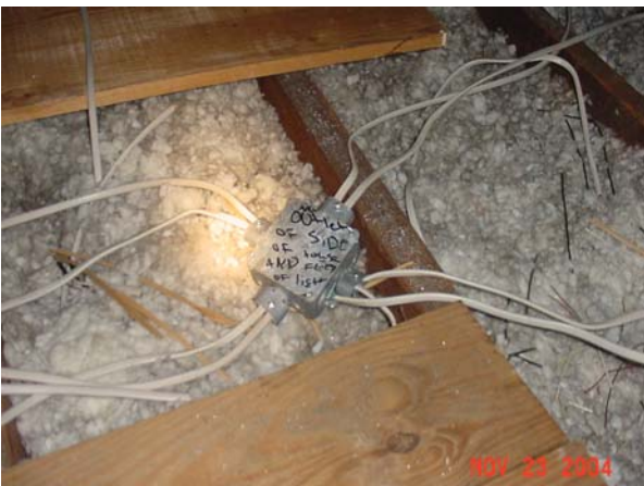
Overfilled Junction Box
