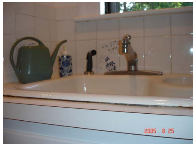
Large gap at sink rim
