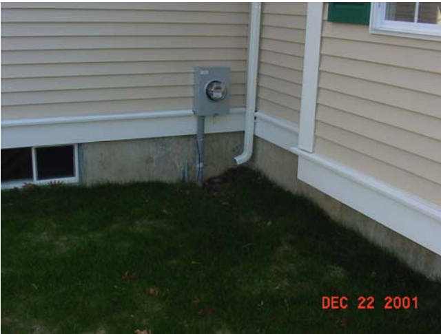
Faulty grading causes wet basements
