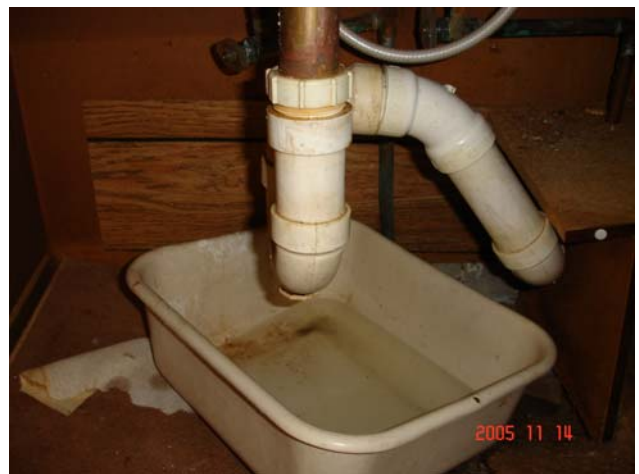
Leaks under sink
