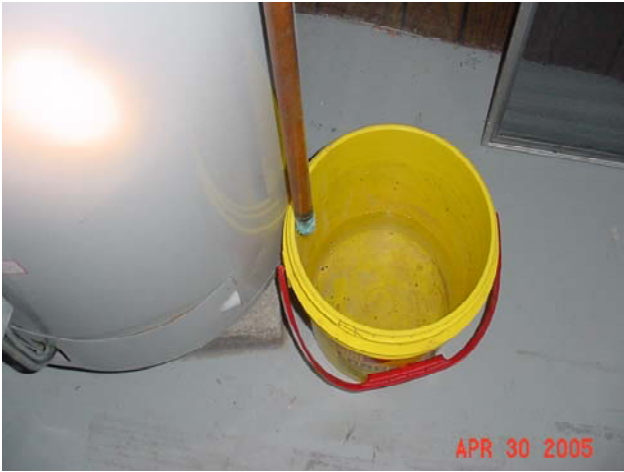
Water heater leaks
