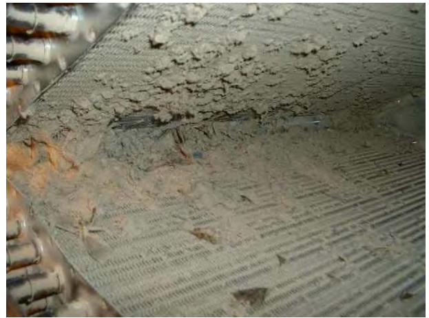
Dirt clogged AC coil
