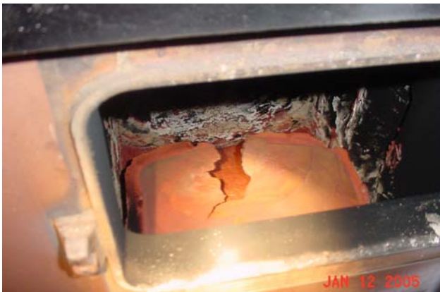
Defective fire chamber
