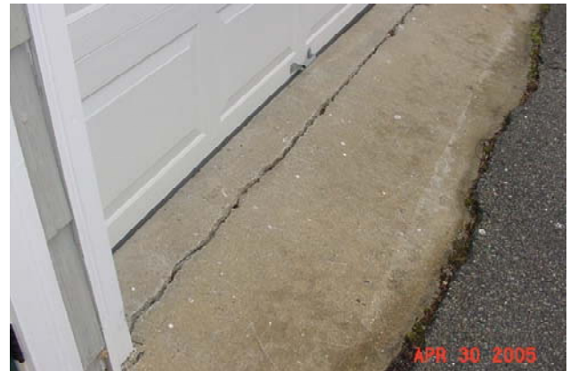
Cracked entry ramp
