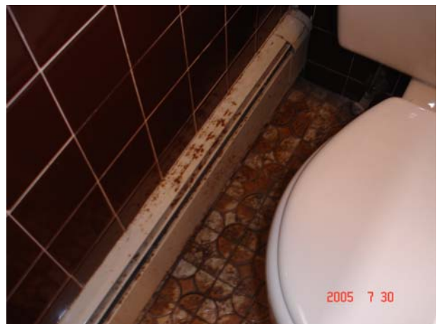
Rusted baseboard heater
