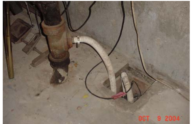
Illegal sump pump discharge
