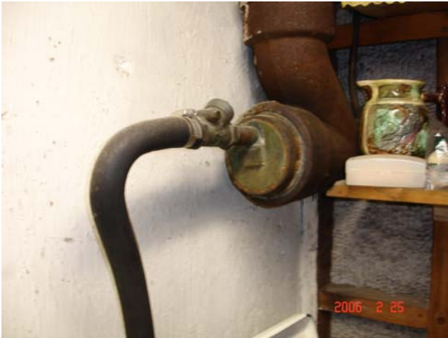
Tampering with the plumbing
