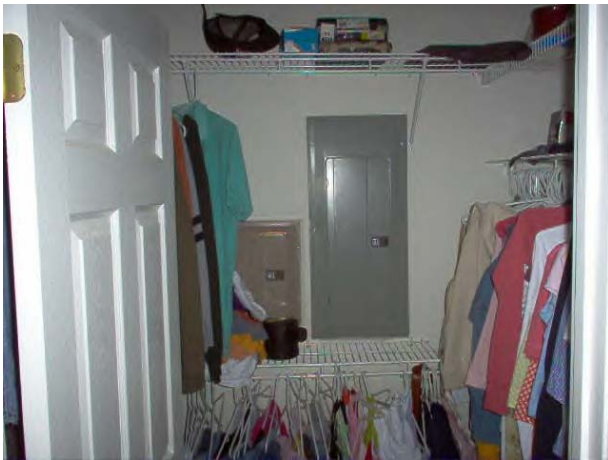
UNSAFE, panel in clothes closet
