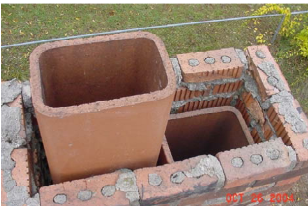
Defective chimney top
