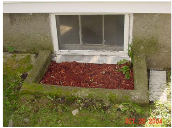
Window well leaks to basement
