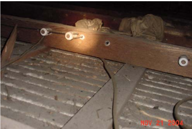
No insulation / old wiring
