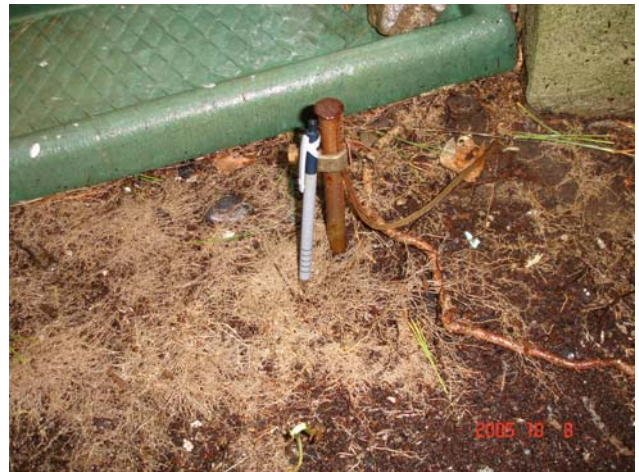
UNSAFE – under driven rod
