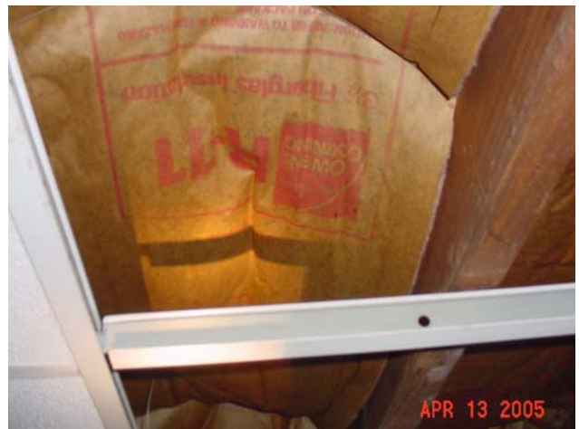
Reversed vapor barrier @ basement ceiling
