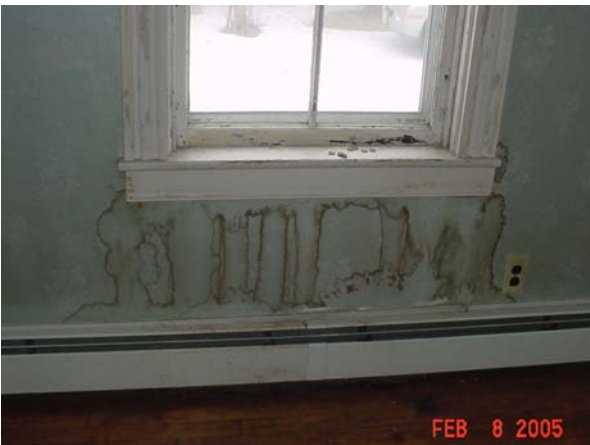
Water stains under window
